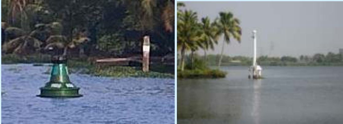
Solar Powered FRP Buoy installed in NW-3 and Beacon lamp in NW-3
